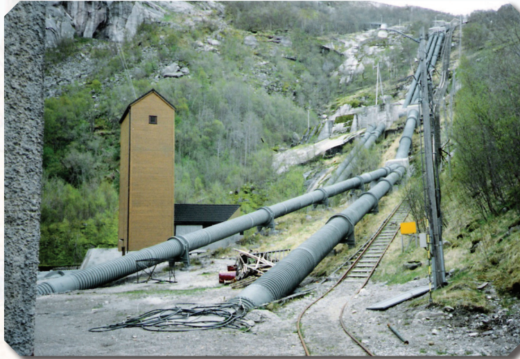
Pipelines to Glomfjord power station.
